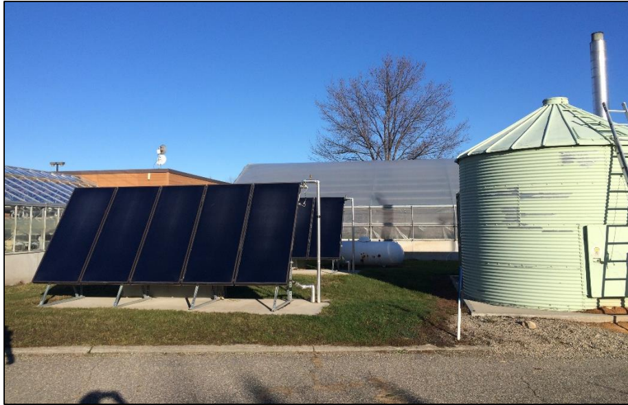
These solar thermal panels are used to heat water for the research centre and the silo contains a furnace that uses local wood-pellets as fuel.
